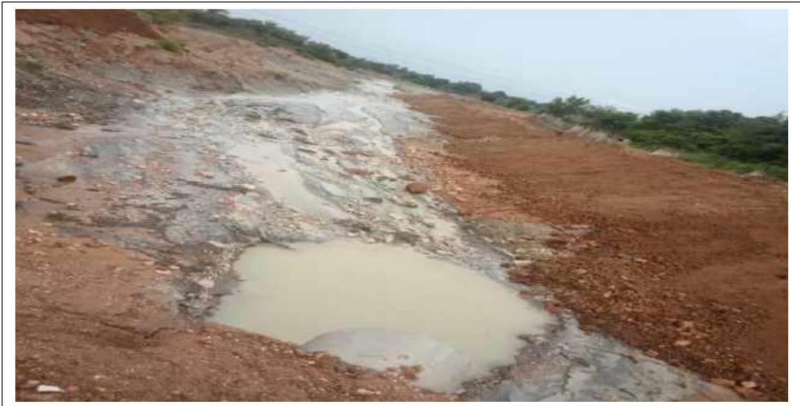
Photograph of the breached site taken on 14.7.2020
