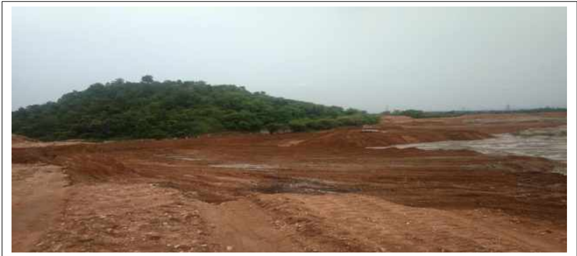
Photograph of the breached site taken on 14.7.2020
