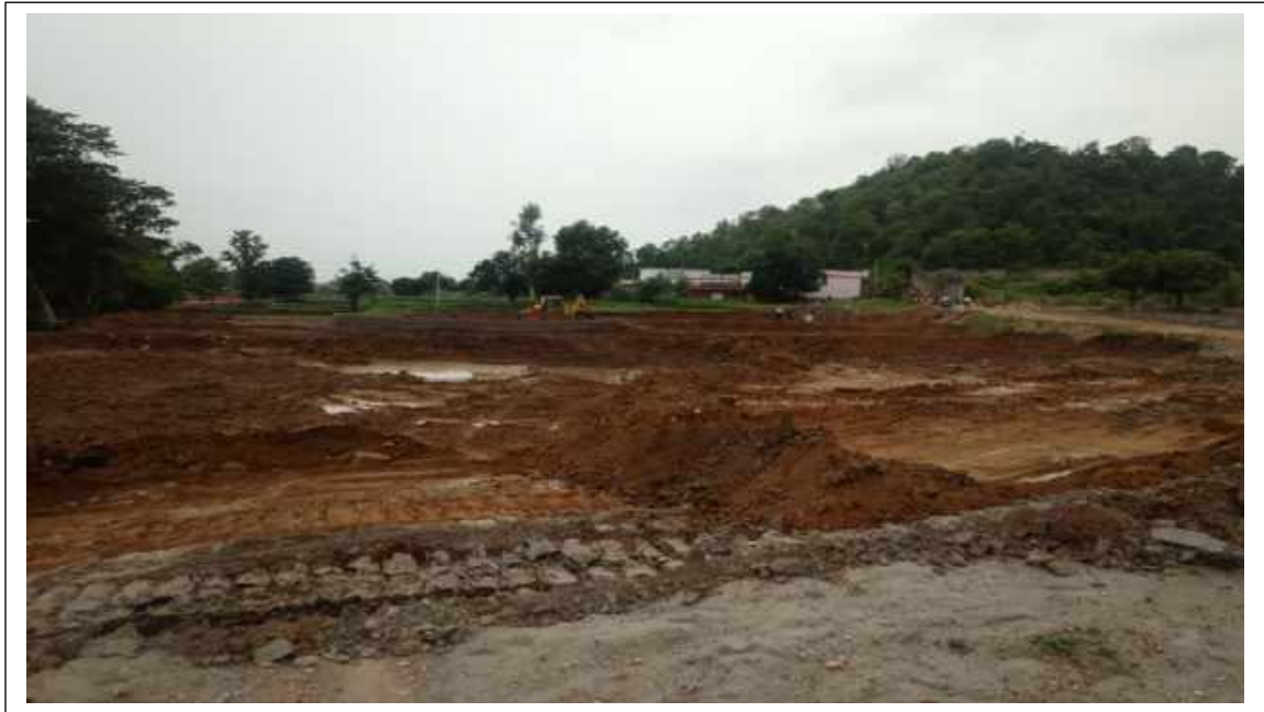
Machineries deployed to restore the ash spread area by collecting the ash and covering the area with soil
